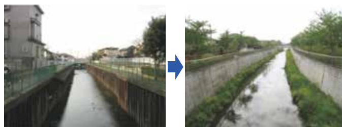
Shakuji River (Before the repair of river walls)
