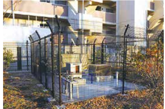
Nakamura Kashiwa Park Emergency Water Well
